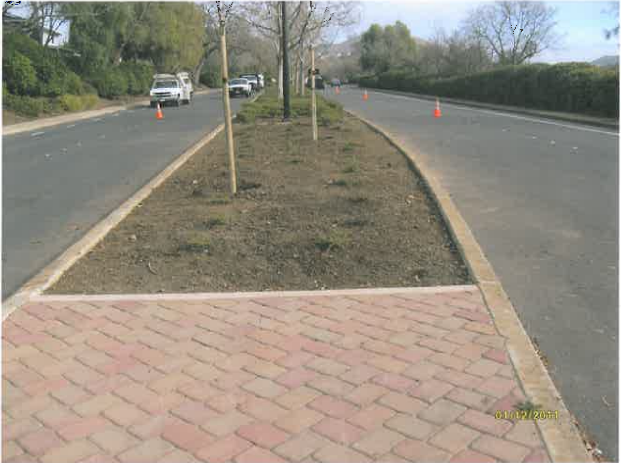
Oakhurst Blvd. -- Yolanda Circle to Eagle Peak completed median: new hardscape/ new infill planting/ new irrigation heads
